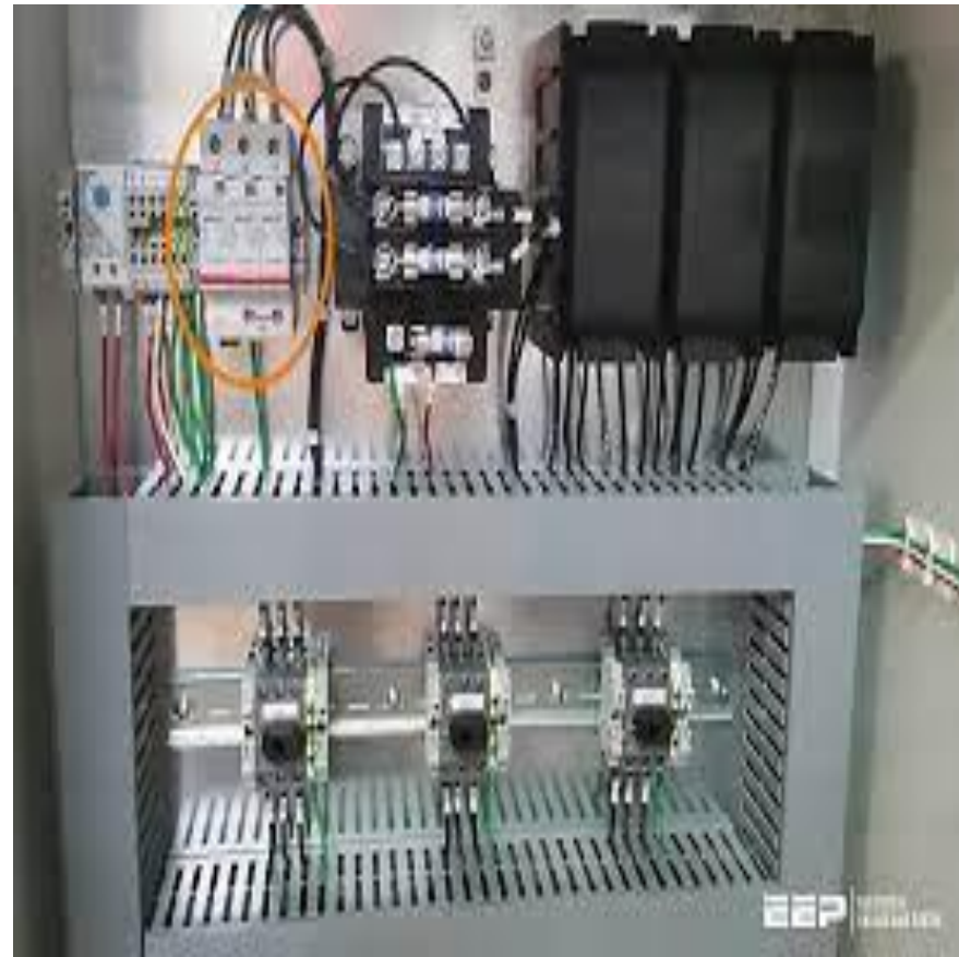
Location at which the surge protector is installed
